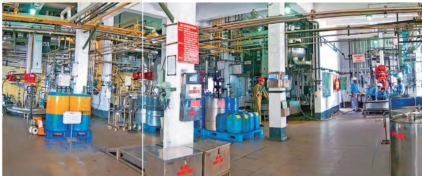
In the API plant, Panoli
