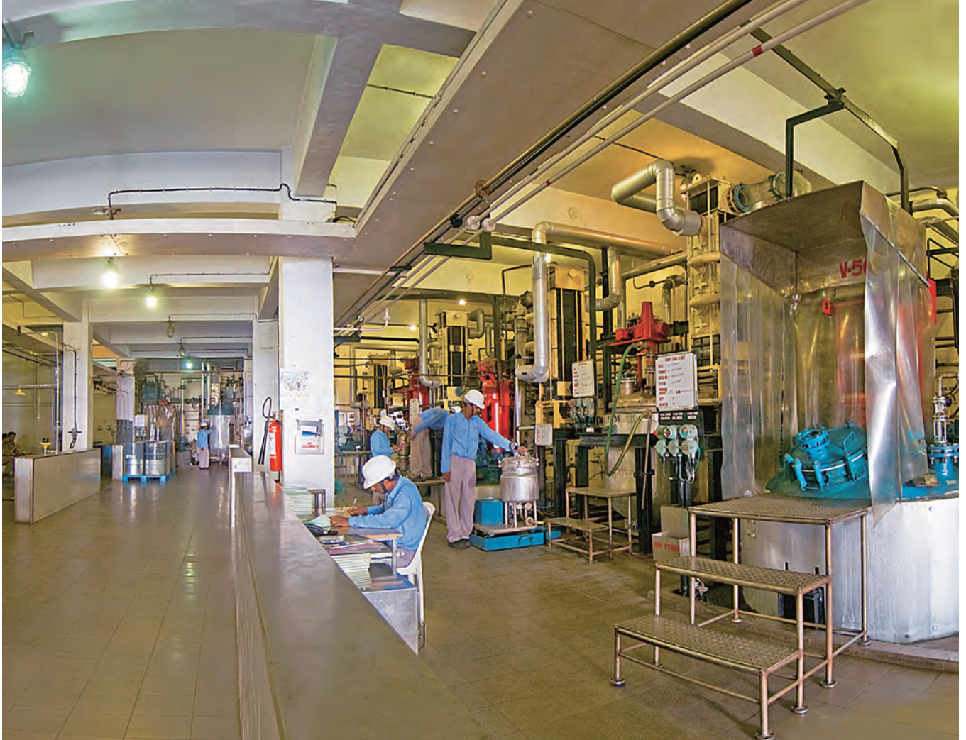
In the API plant, Ahmednagar
